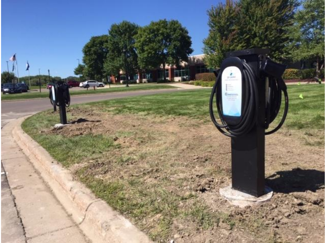
WH recently installed six ZEF Energy chargers in their parking lot to prepare for future EV use by employees.
